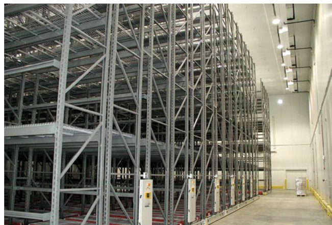
Offering the industry's leading applications expertise, our storage solutions specialists can design and implement a mobilized storage system like the above for your specialized applications.
