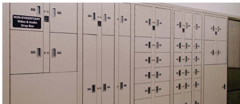
Multiple rows of Locker configuration 15 with full size refrigerators along the back wall at Wake County Detention Center
